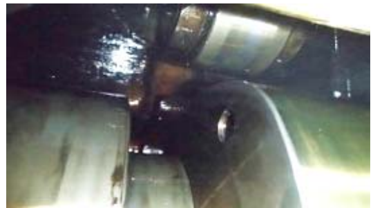
写真-5 Pump Roller no contact Photo-5 Pump Roller no contact
